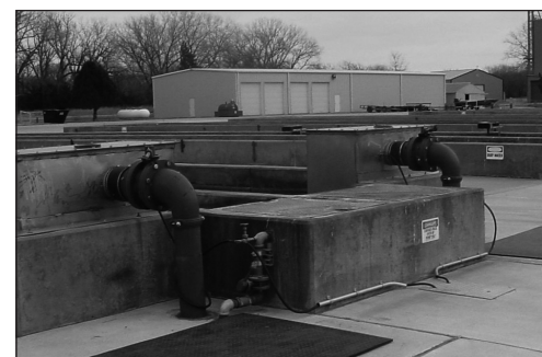
RW Aeration Chamber
